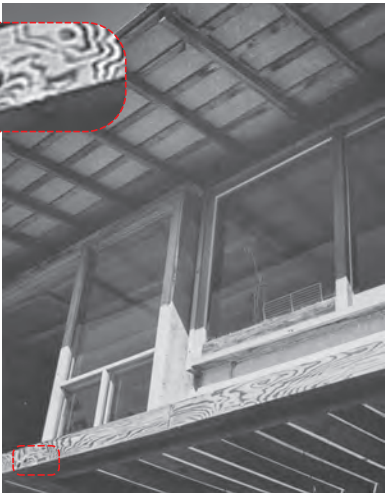
Figure 16.6 | The detail view of this image shows the heads of bolts that likely connected the band board with joists behind, ca. 1952 (Source: Nakashima Foundation for Peace).
