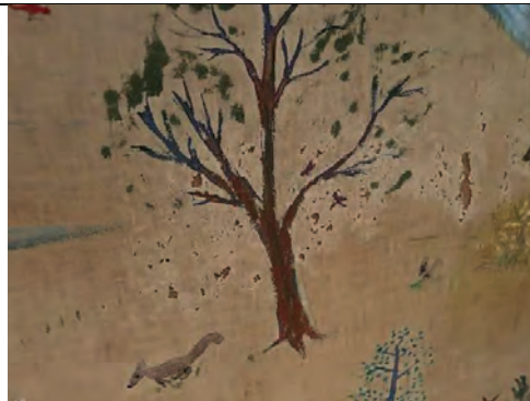
Fig.3.13 NFH office bedroom: suspected silverfish damage to Mira Nakashima mural Photo credit: Wendy C. Jessup October 2023
