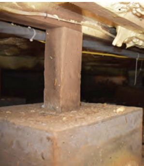
Figure 14.7 | A foundation post secured to the concrete footing with no visible connectors (Source: CAC, June 2024).
