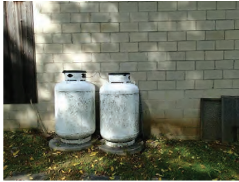
Fig. 2.59 Fuel Supply for Emergency Generator Photo credit: Michael C. Henry October 2023
