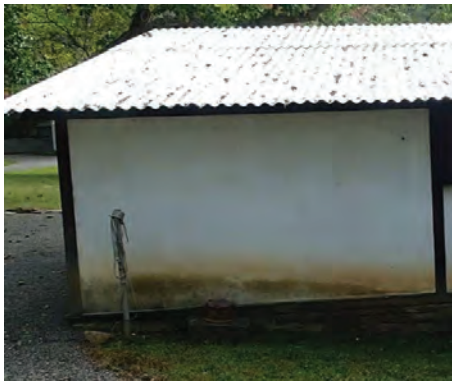
Fig. 2.41 Water damage to Garage wall Photo credit: Michael C. Henry October 2023
