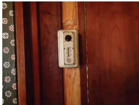
Fig. 2.48 Thermostat for fan coil unit in Parents' Bedroom Photo credit: Michael C. Henry October 2023
