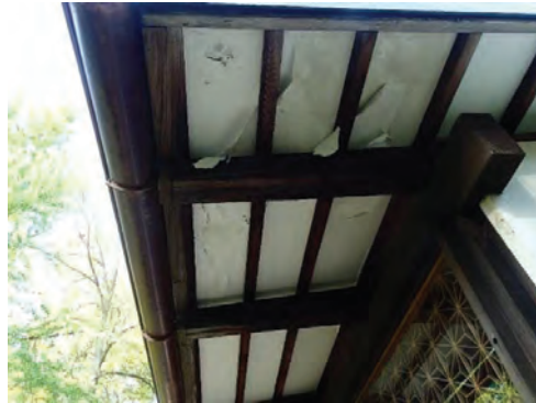
Fig. 2.40 Gutter on 1954 second build may damage soffit Photo credit: Michael C. Henry October 2023
