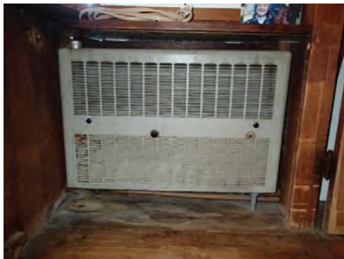
Fig. 2.47 Hot water fan coil unit in Parents' Bedroom Photo credit: Michael C. Henry October 2023
