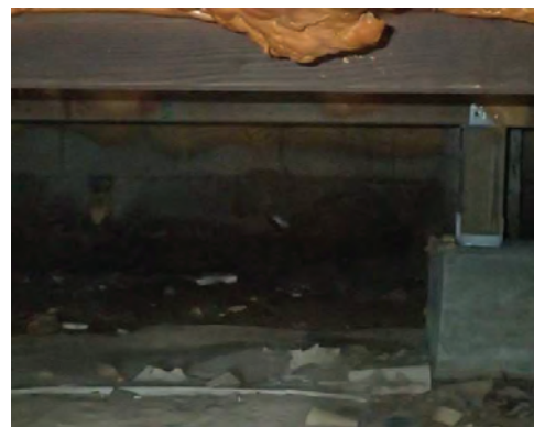
Fig. 2.44 Past and active rising damp on CMU in crawl space Photo credit: Michael C. Henry October 2023
