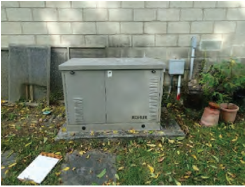
Fig. 2.57 Emergency Generator Photo credit: Michael C. Henry October 2023
